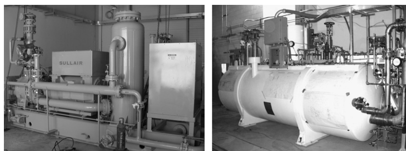
Fig. 7. 7.5 kW helium refrigeration system compressor (left) and cold box (right).
